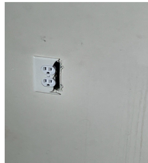
Issue #3- Outlet cover is broken
