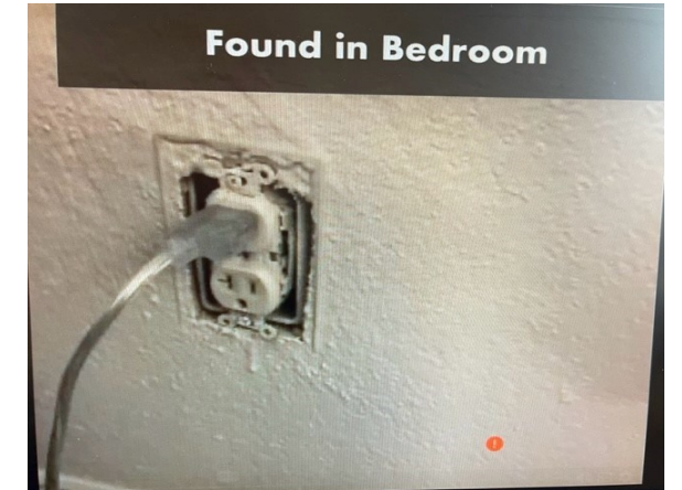
Issue #2- Outlet cover is missing
