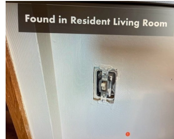
Issue #1- Switch cover is missing
